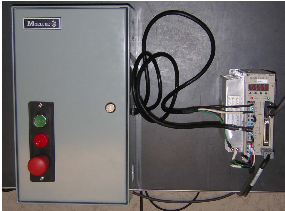
Figure 71: Wiring between amplifier and starter
