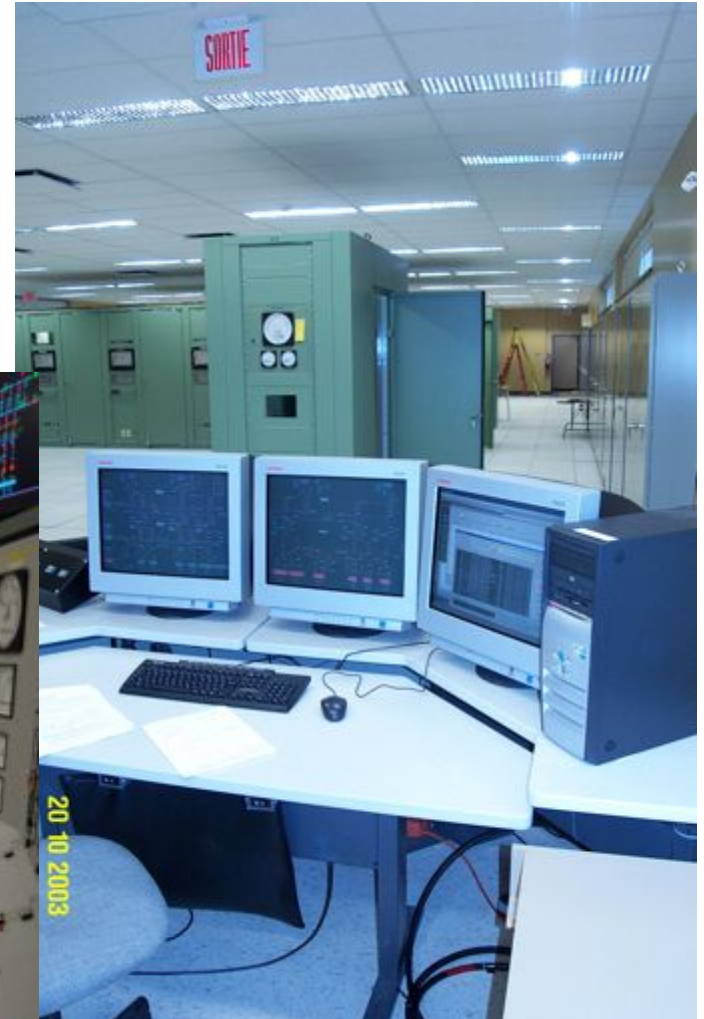
Boucherville substation HMI
